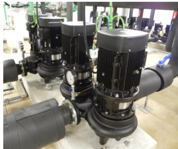
Grundfos TPD twin pumps used in a medium size chilled water plant
