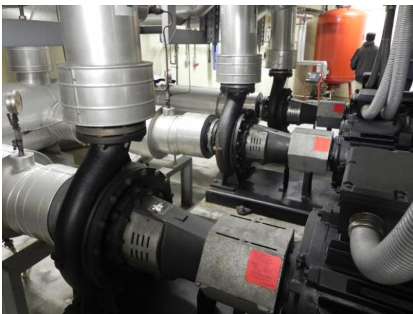
Secondary pumps in a large stadium chilled water plant
